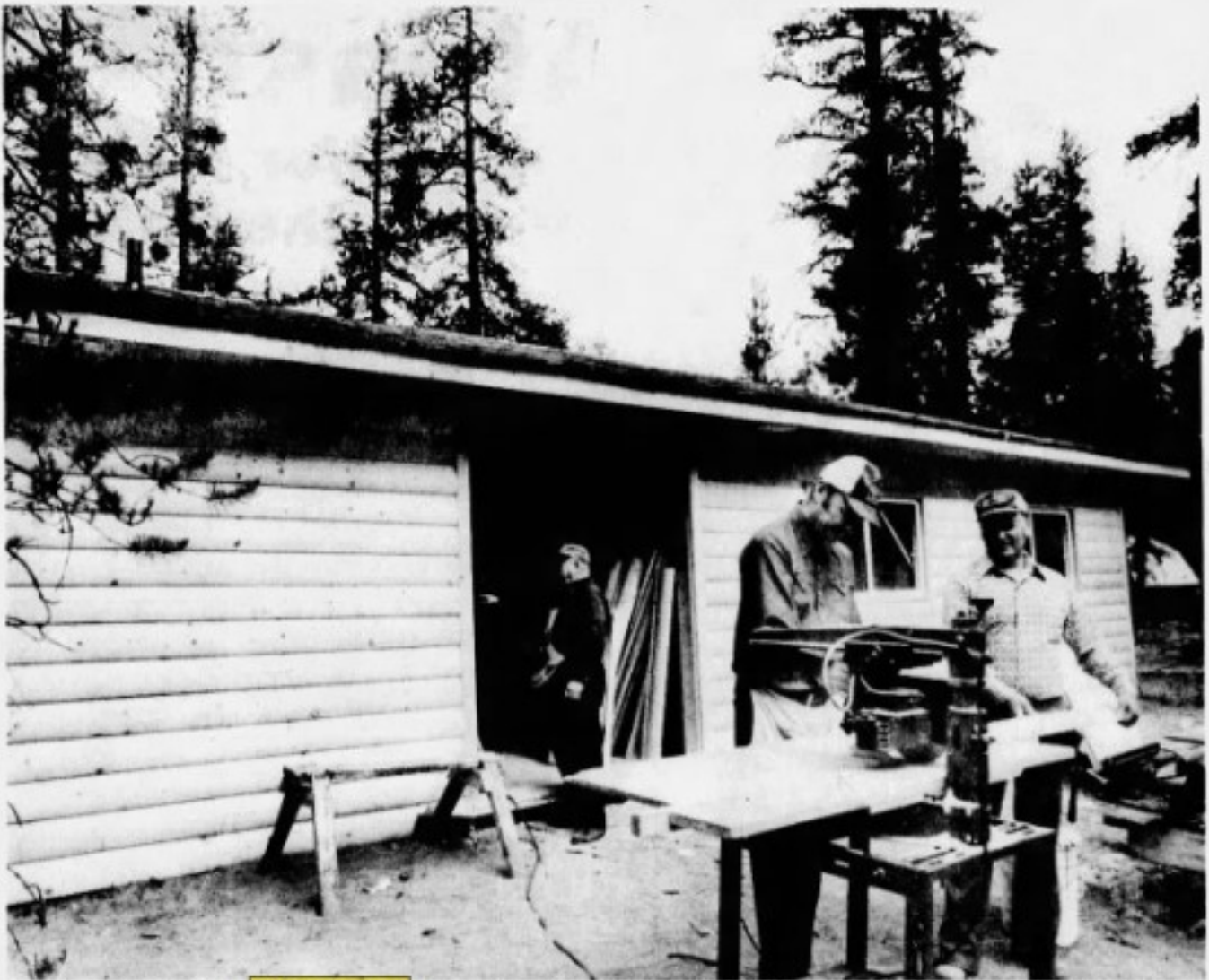
Charlie Wales (left) and Ritchie McRae handle the sawing chores while Bob Rycroft Sr. wields a paint brush as a rest area of the new fairgrounds takes shape.
